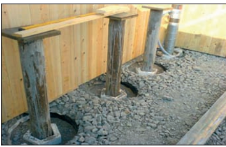
Fig. 5: Piles have been driven. The pile to the right was later used for monitoring. The picture shows the loose sand and styrofoam plates that were used to achieve a less stiff surrounding for the upper part of the piles
